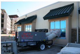
A 7.5-ton Comfort-on-the-Run portable air unit was used in the chapel for the contractor to work on finishes
