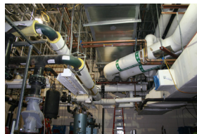
HVAC piping and ductwork in the Domiciliary
