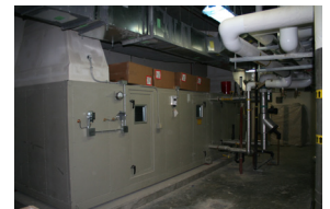
One of four mechanical rooms housing a 25-ton AHU in the Domiciliary
